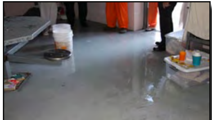
The inmates had to take shifts emptying the buckets when it rained because of major water leaks in the jail facility.
